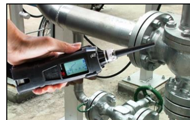
For gas pipe joint
